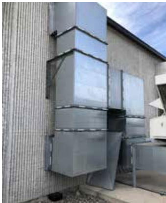
Existing AAON RTUs duct work
