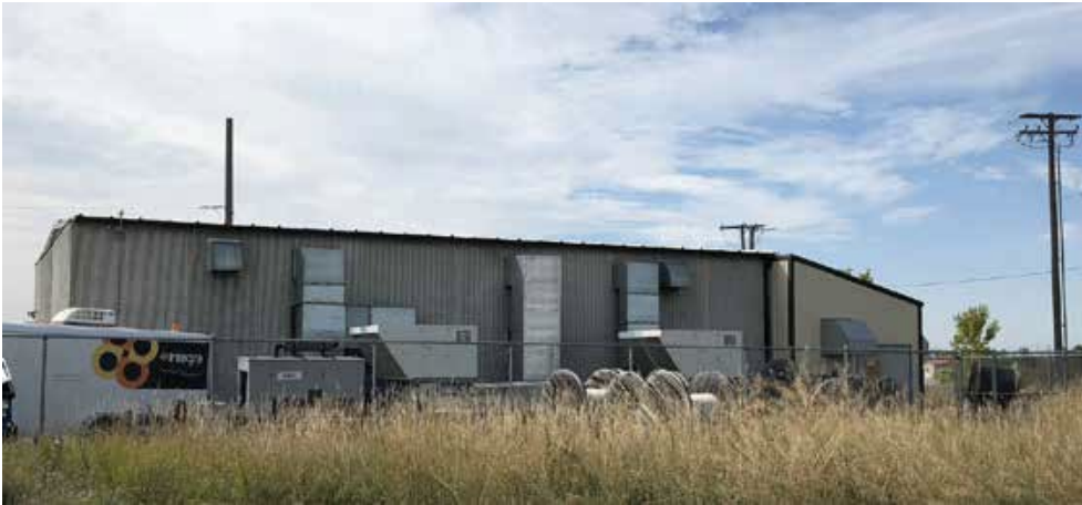
Two AAON RTUs ducted into facility from north side of shelter
