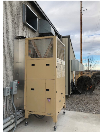
Exterior pad and duct work connections
