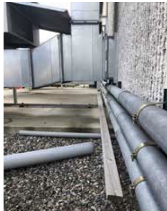
Existing AAON RTUs duct work
