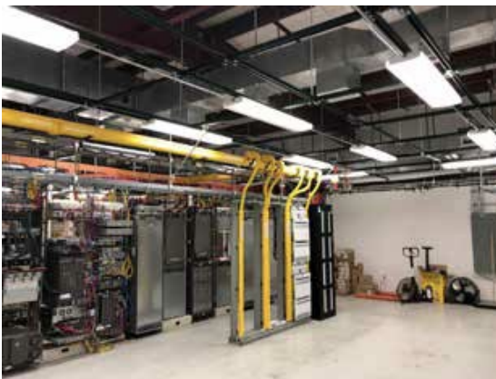
Extensive duct work throughout the facility
