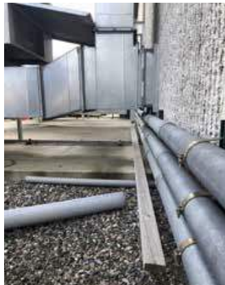
Existing AAON RTUs duct work
