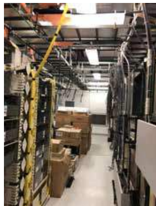
Rack systems and IT equipment
