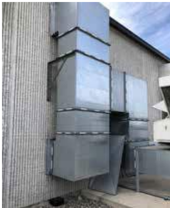
Existing AAON RTUs duct work
