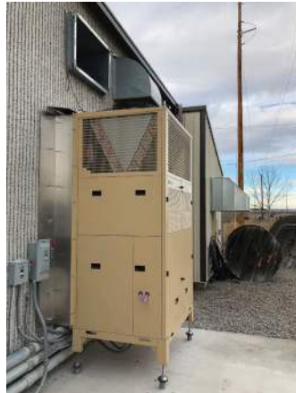
Exterior pad and duct work connections
