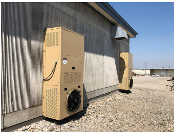
East Side of Helena Data Center
