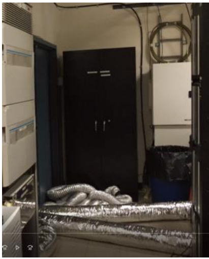
Supply air ducting for the IT racks
