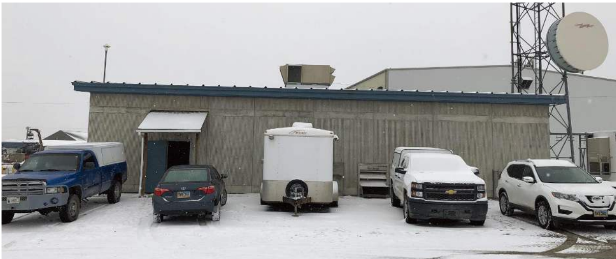
Front entrance with the Lennox Roof Top Unit (RTU) installed in the middle of the structure
