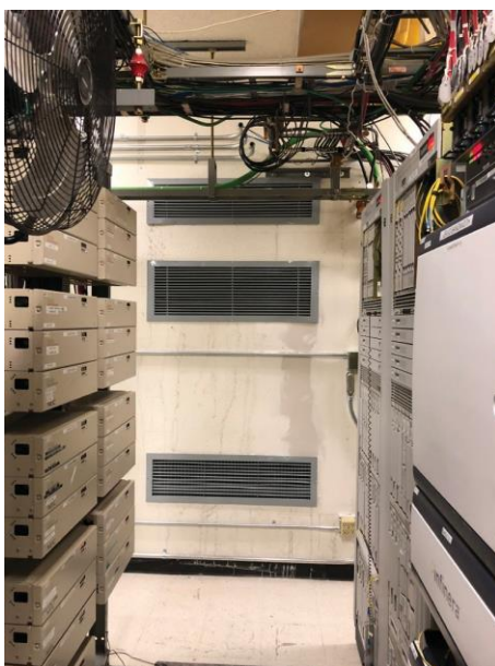
Interior shot of Unit 3 grills
