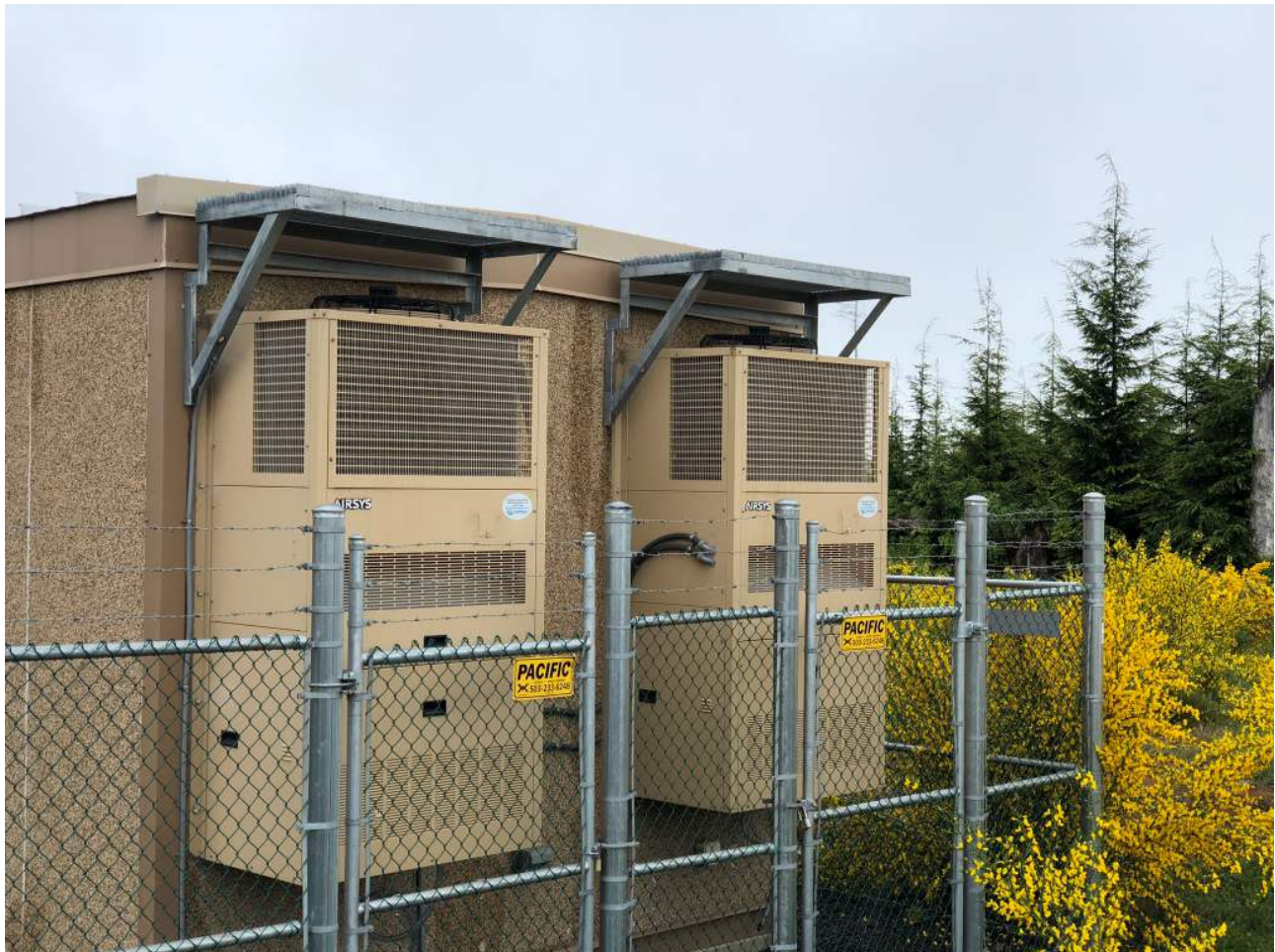
Two Unit AIRSYS UNICOOL system installation at a telecom shelter located in Astoria, OR
