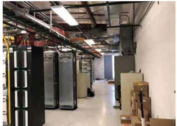
Existing Liebert Challenger Units (against the wall in dark grey)
