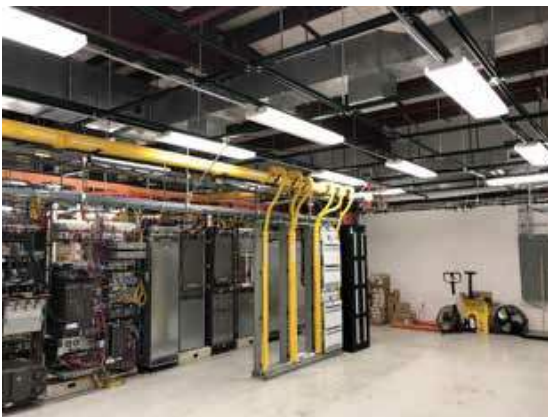
Extensive duct work throughout the facility
